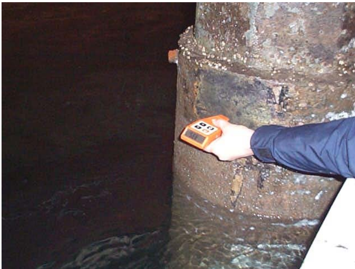
Plate 3. Thickness Readings of Galvanising to Collars
